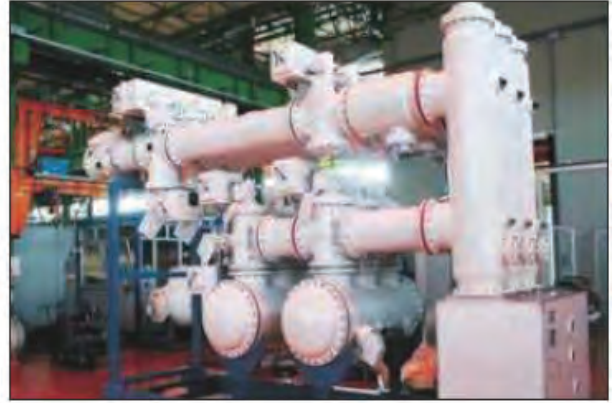
170kV GIS : 3-Ph Enclosed Busbar
